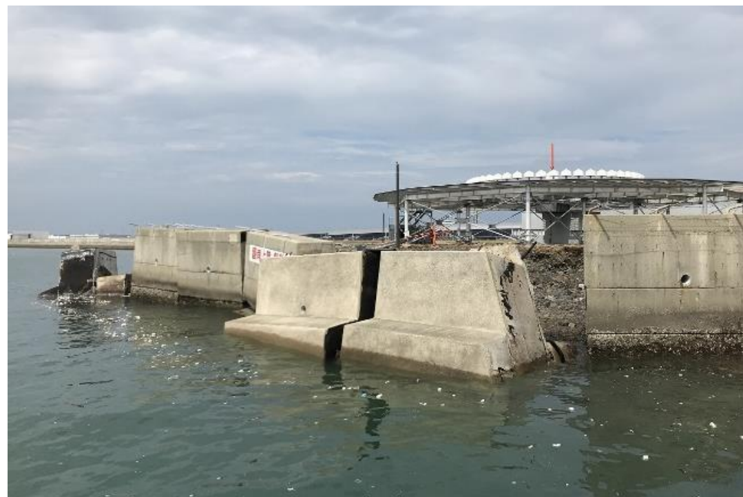
< Collapse section at Kansai Airport >
